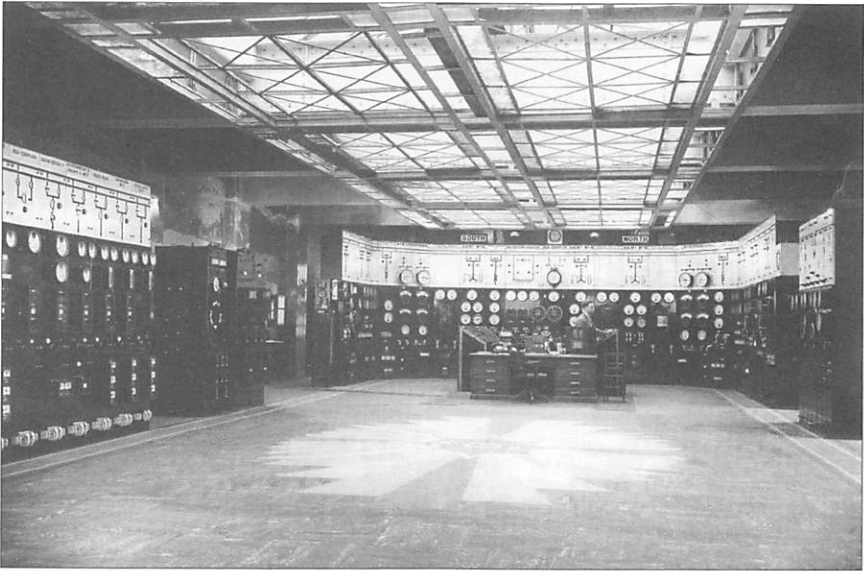
Fig 5 Control Room, Croydon Power Station. This station became known as Croydon 'A' when Croydon 'B' power station was built after the Second World War. Courtesy of Amberley Working Museum.
