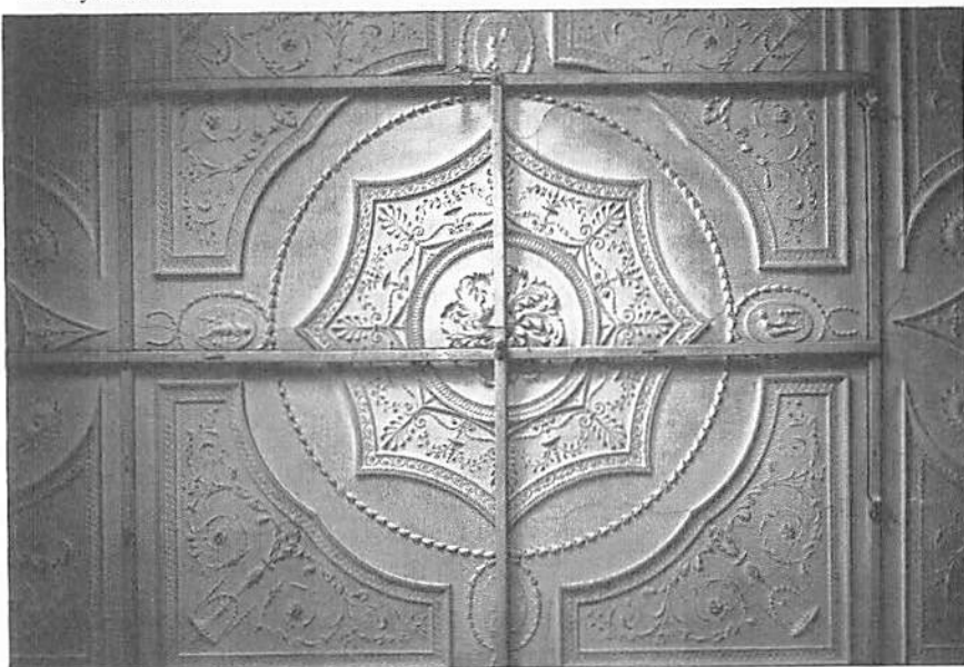
Fig. 5 Ceiling of the Drawing Room added to Shalford House in 1797 from a photograph held by the NMR.
