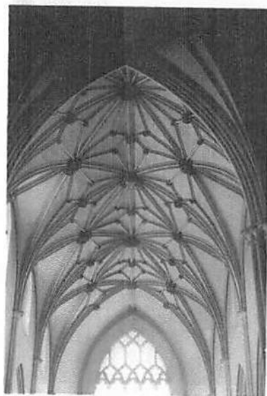
Fig. 4. Mitcham Church: The plaster vault of the nave seen from the chancel.
