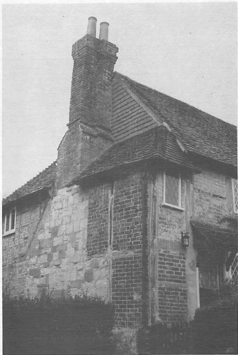
3. Firestone in chimney at Church Lane Cottage, Godstone.
