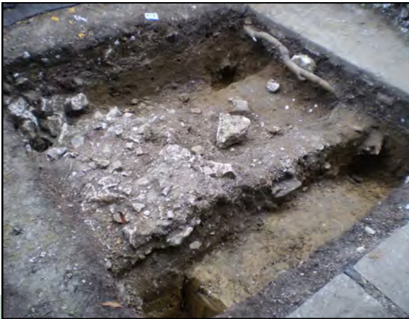
Figure 4 Trench 8 with demolition material between partially robbed out walls. In the photo the near slot has removed the wall foundation.
