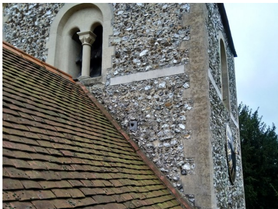
Fig 8 Tower east side showing slight overlap of nave roof on belfry opening
