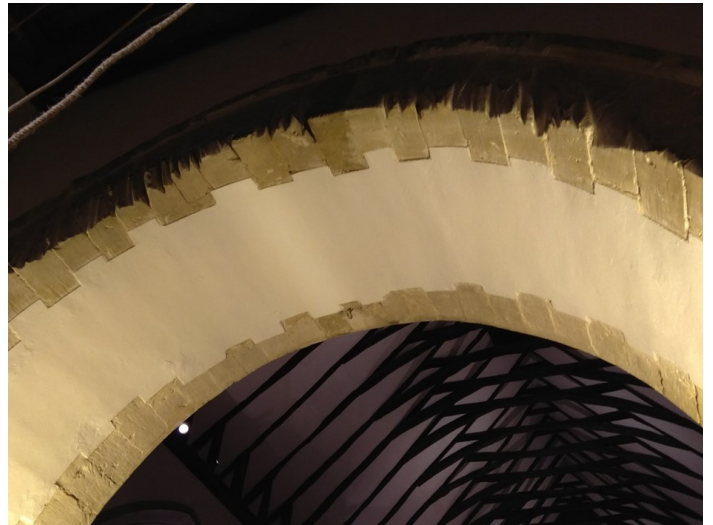
Fig 6 Interior of tower arch showing deep grooves
