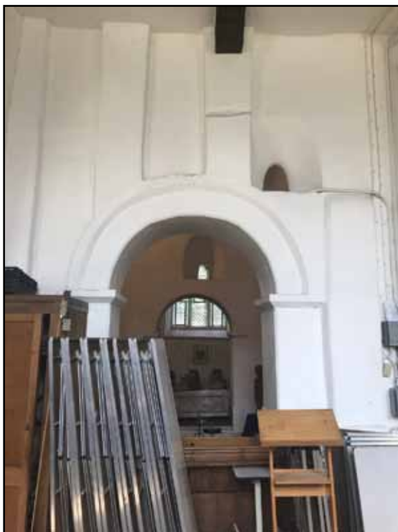
Figure 3: Interior view of the lowest levels of the south face of St Mary's tower, showing original pilasters and double-splayed window, with another visible through the later, probably late 11th/early 12th-century transept arch.
