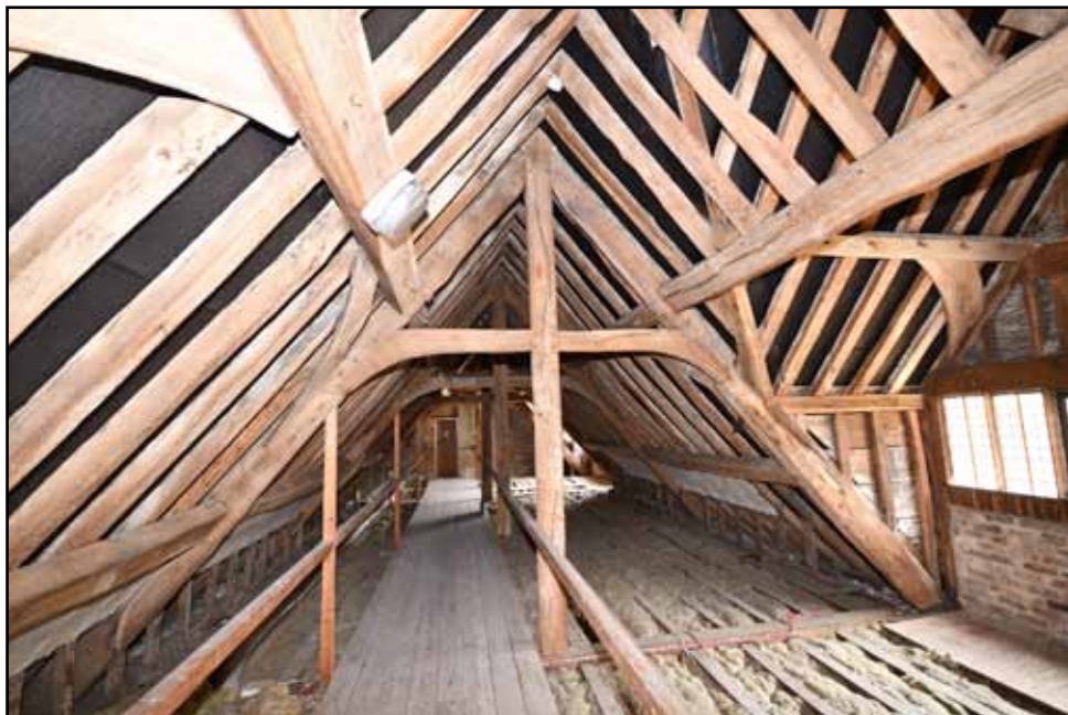
Kingposts in the roof over the East range of the outer court, Lacock Abbey
